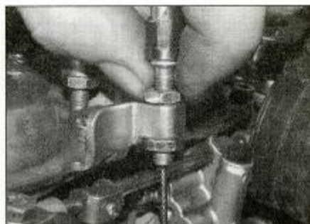
16.6c Draw the cable up so the bottom nut is captive against the bracket, then tighten the top nut
