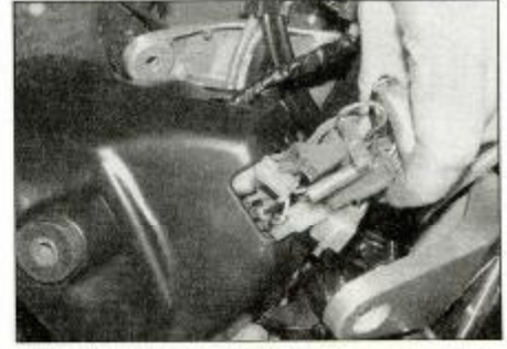
8.4c . . . then remove the shell and feed the wiring connectors out the back
